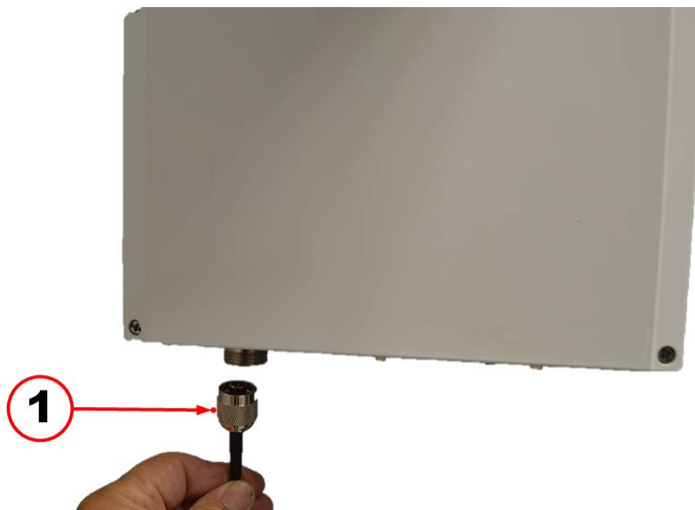
Figure 94 RF Filer to CGR Connection
