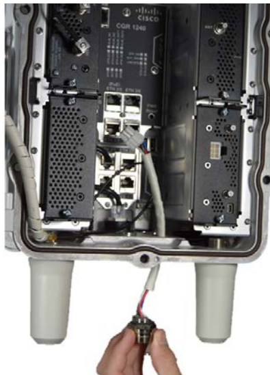
Figure 52 PLC Signal Cable and Cable Gland Location
