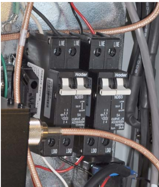
Figure 6: On/Off Circuit breakers.
