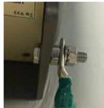
Figure 59 Remote Ground Connection
