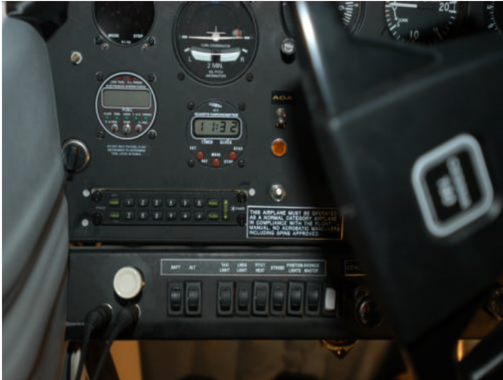
PTA-12 Dialer Install Location
