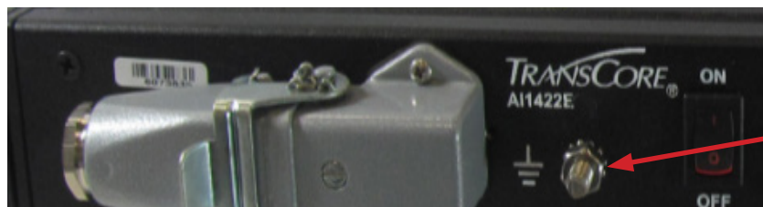
Figure 24 Location of Ground Stud
