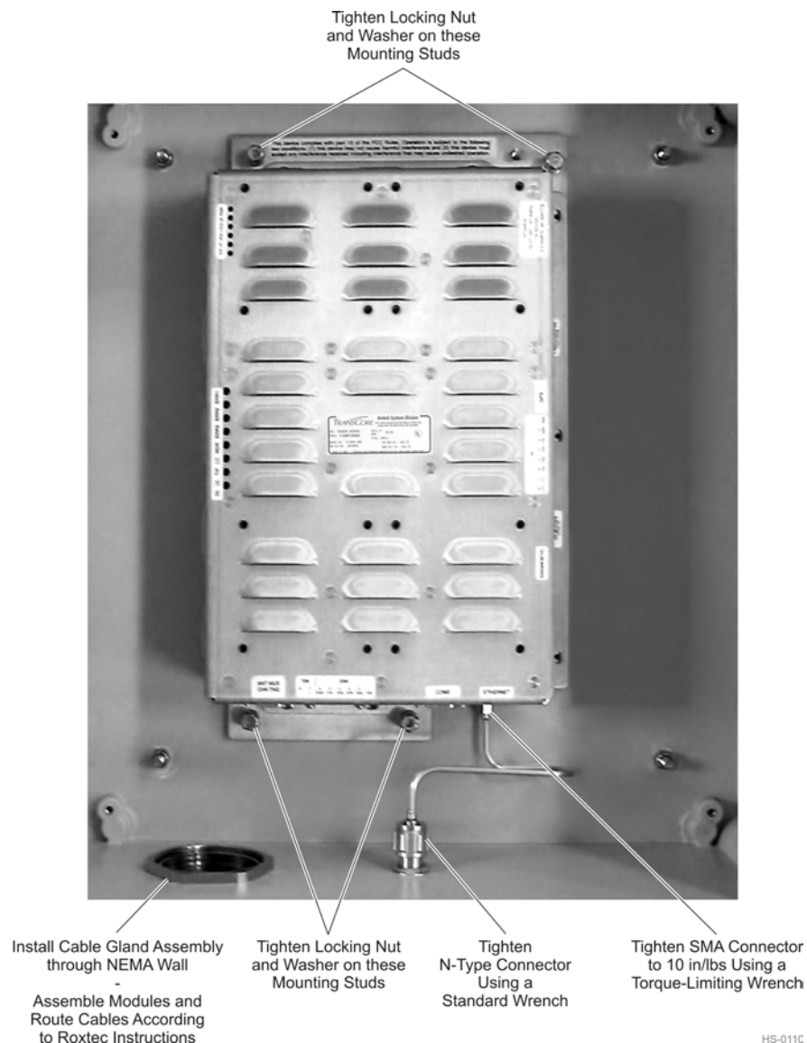
Figure 3-9 Encompass Reader Mounted in a NEMA Enclosure
