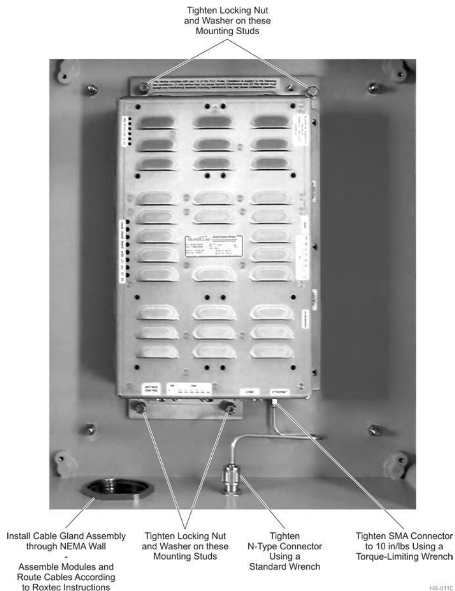
Figure 3-9 Encompass Reader Mounted in a NEMA Enclosure
