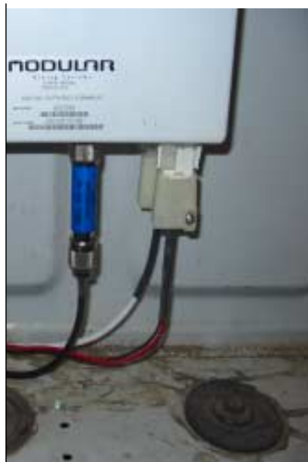
Figure 2.24 Cable 302202 Attached to Attenuator
