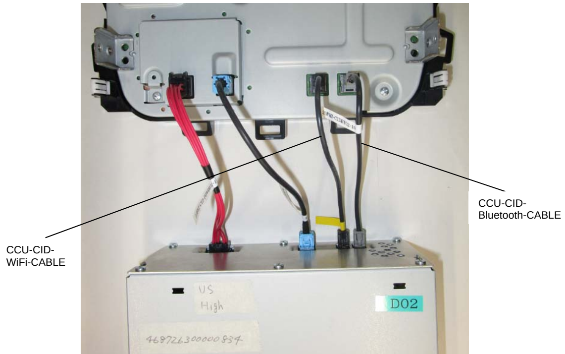
Connection part of the CCU and CID
