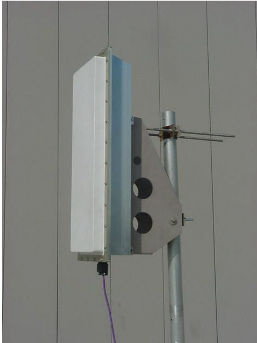
Figure 3-3: Base Station ODU
