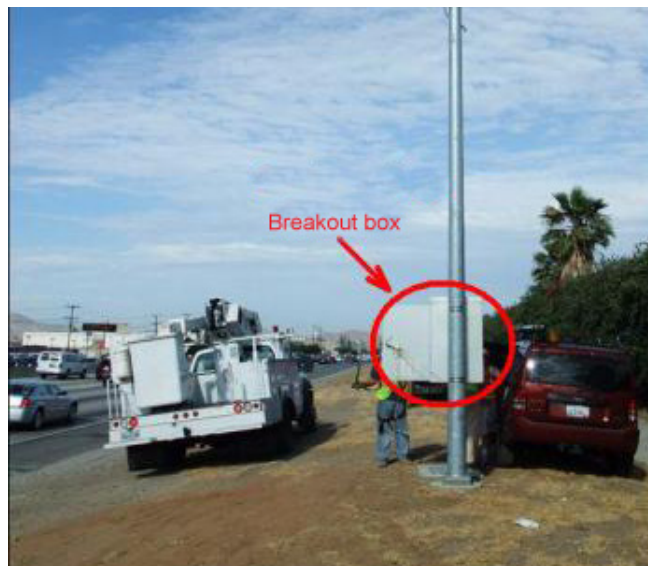
Figure 2-3: Typical Breakout Box Installation
