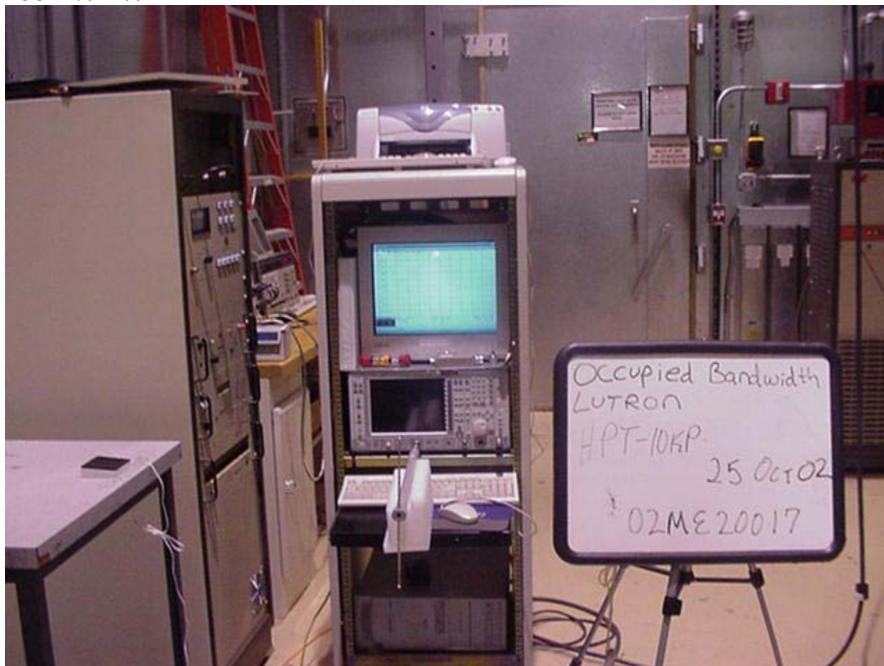
Occupied Bandwidth Test Set-Up HRT-10KP
