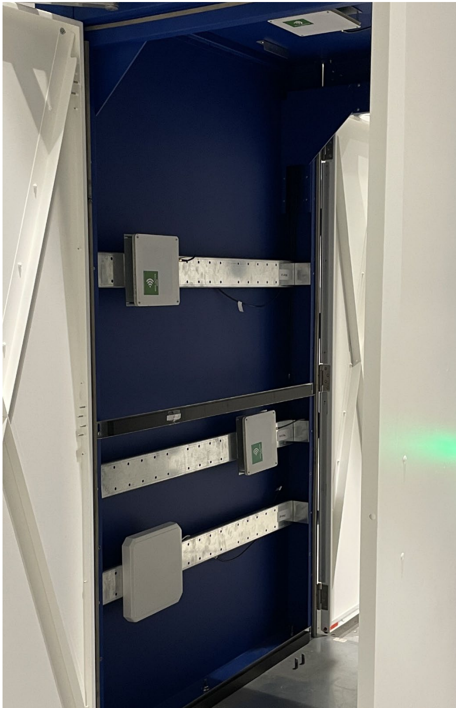
View of antenna mounting, right side
