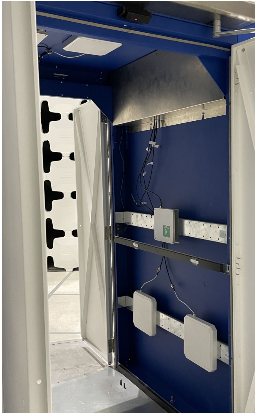
View of antenna mounting, left side
