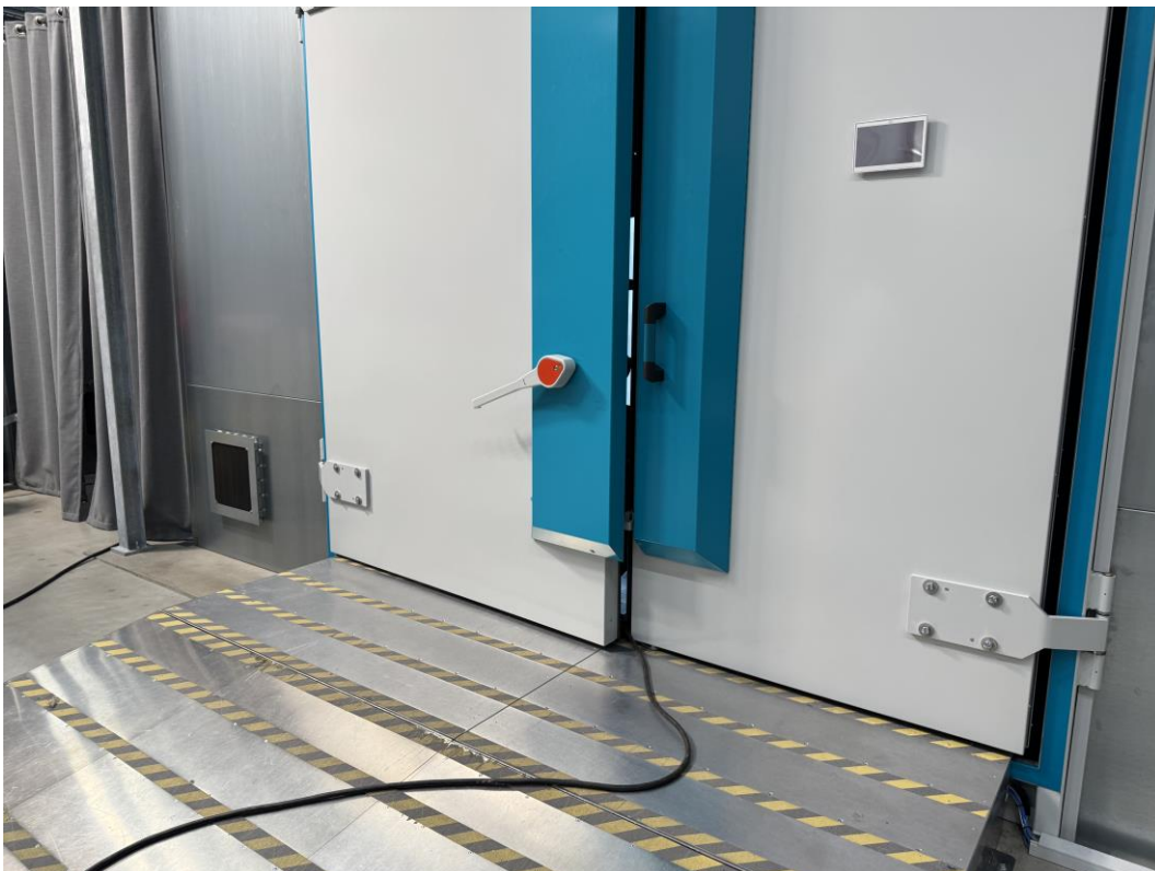
Photograph 6: Overall view. Power supply cable going through the door in the chamber.
