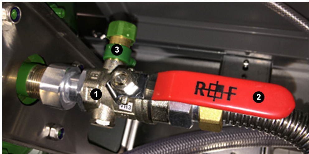
Figure 4-48: Valves VH3 and VS3 on pump unit 40 l/min); valves VH5 and VS5 on pump unit 80 l/min
