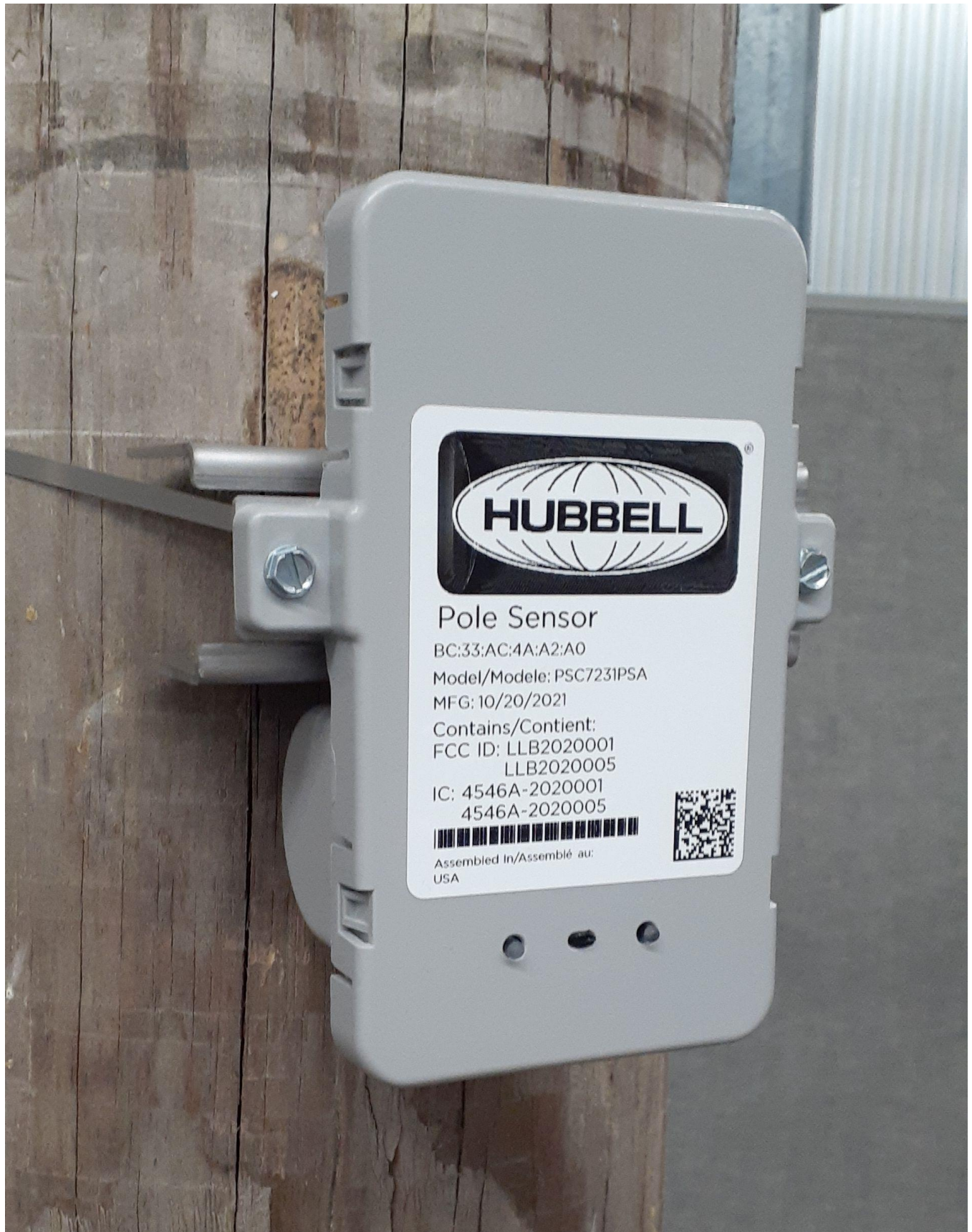
Pole Sensor installed
