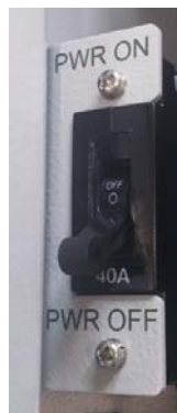
Figure 3-29 HPR AC Switch
