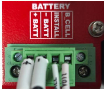
Figure 3-6 Battery Backup Terminal Block
