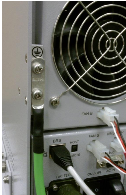
Figure 22 Ground Cable Connection
