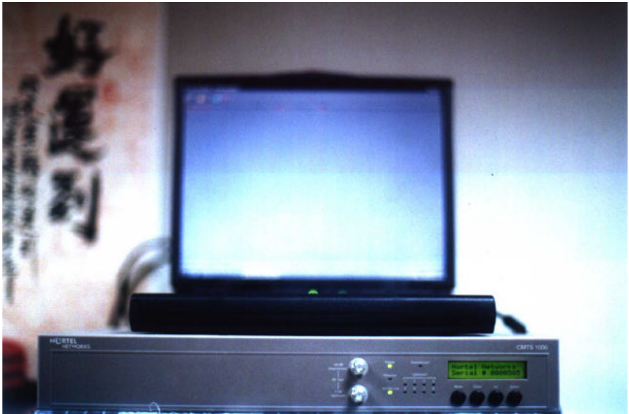
Cable Modem Head End
