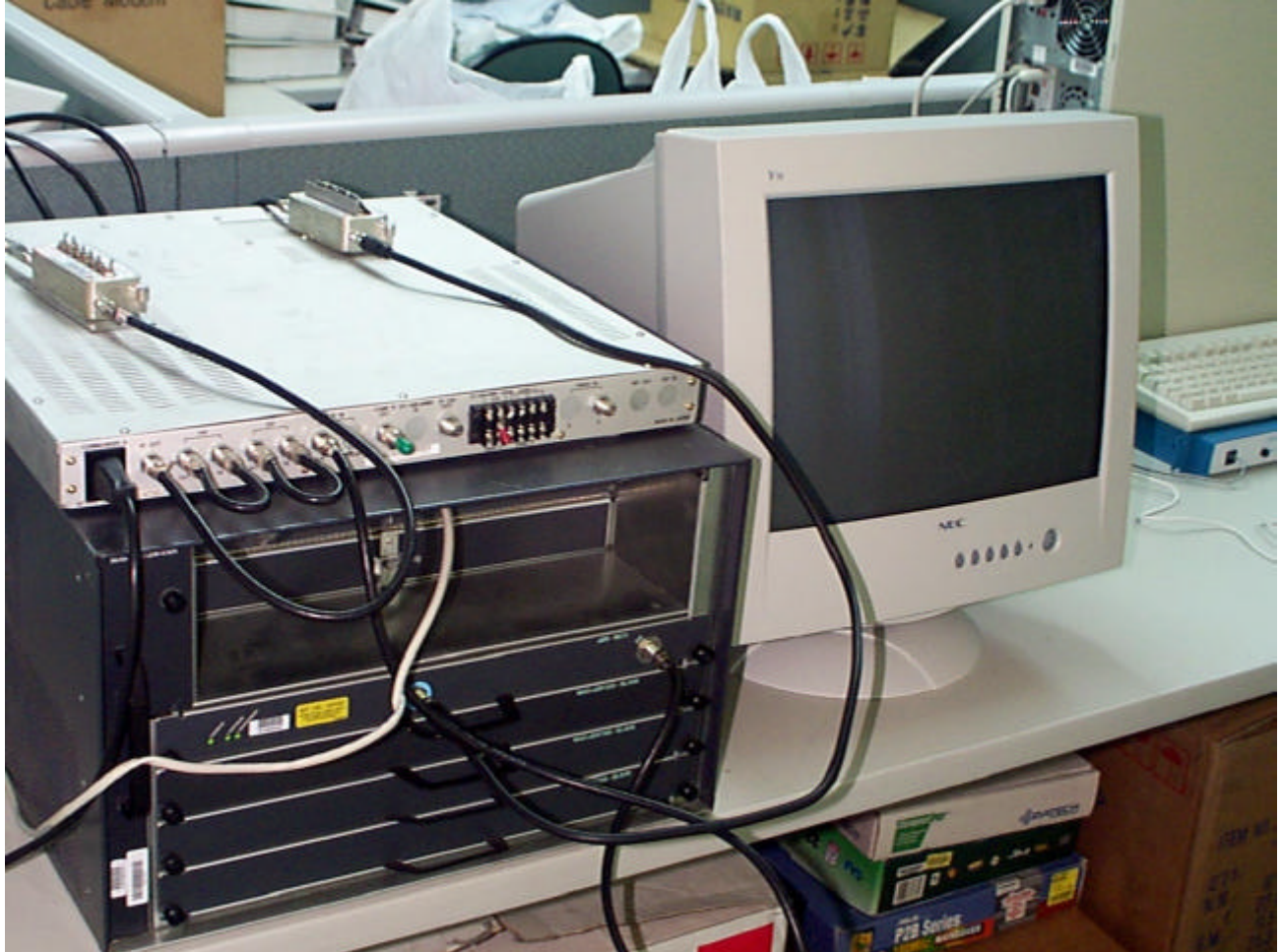
Cable Modem Head End
