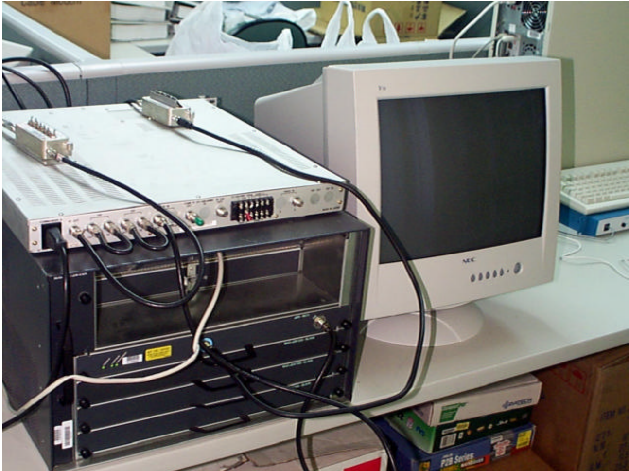
Cable Modem Head End
