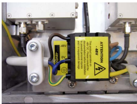
Figure 3-35: -48VDC Power Connections
