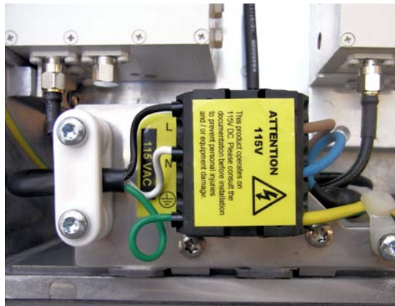
Figure 3-34: 115VAC Power Connections
