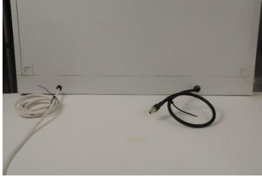
RF Cable Inserted into Cabinet
