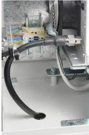
RF Cable Connection
