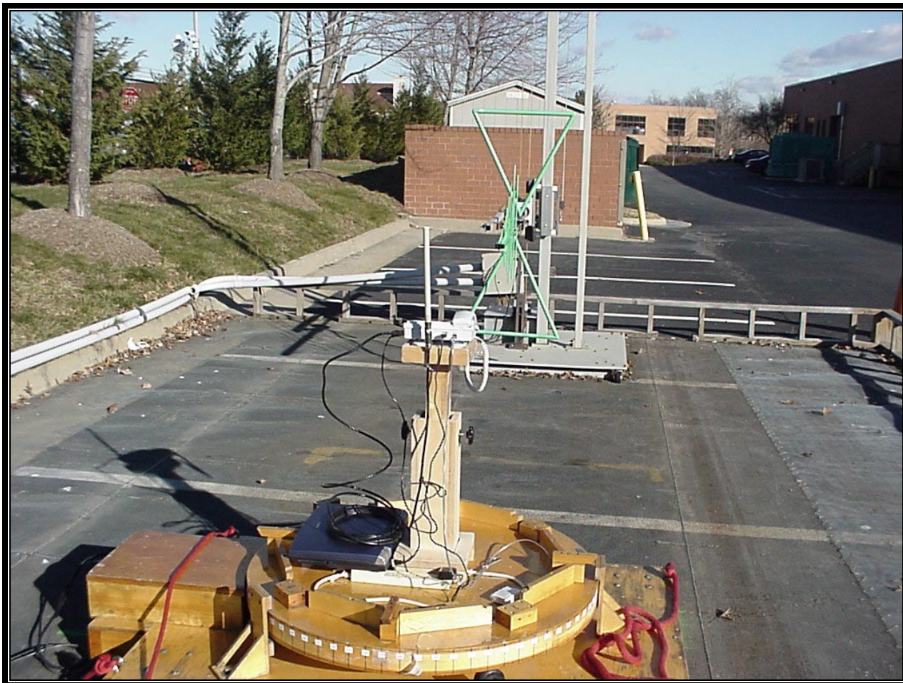
PHOTOGRAPH 7: RADIATED BACK VIEW WITH ROD ANTENNA
