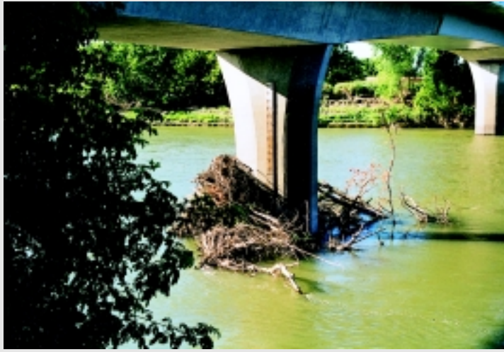
River with debris
