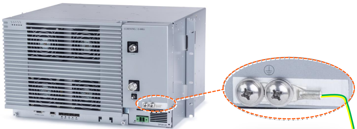
Figure 7MRU Grounding Lug
