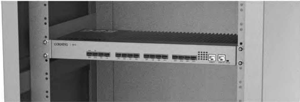
Figure 18. E3 in Rack
