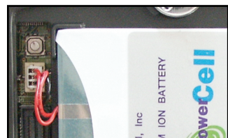
Battery Cable Plugged In
