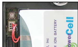
Battery Cable Plugged In
