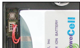
Battery Cable Plugged In
