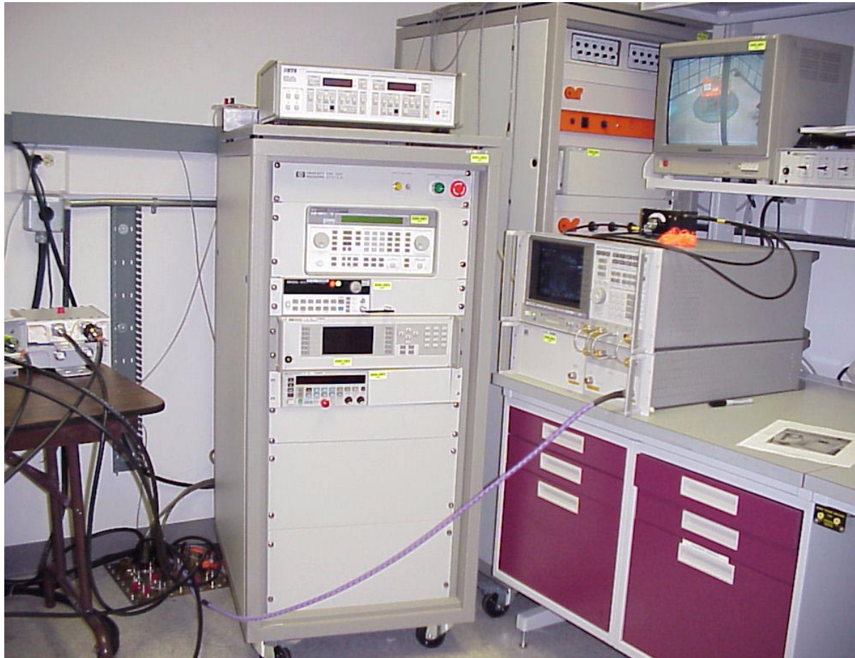
Figure 12.7 3-Meter Control Room
