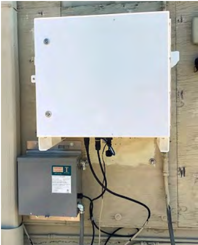
Figure 18 – RMDC Mounted on Wall
