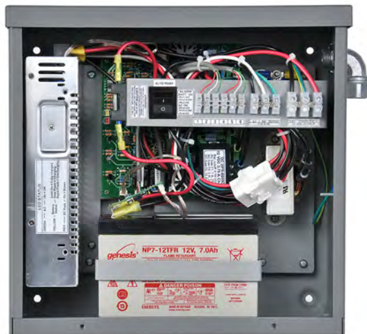
Figure 36 – Outdoor UPS (Cover Removed)
