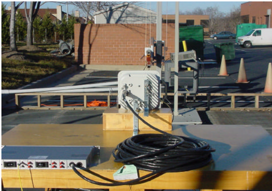
PHOTOGRAPH 7: CONFIGURATION OF TESTED SYSTEM (FRONT VIEW) HORN
