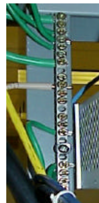
Detail of Equipment Rack Ground Block
