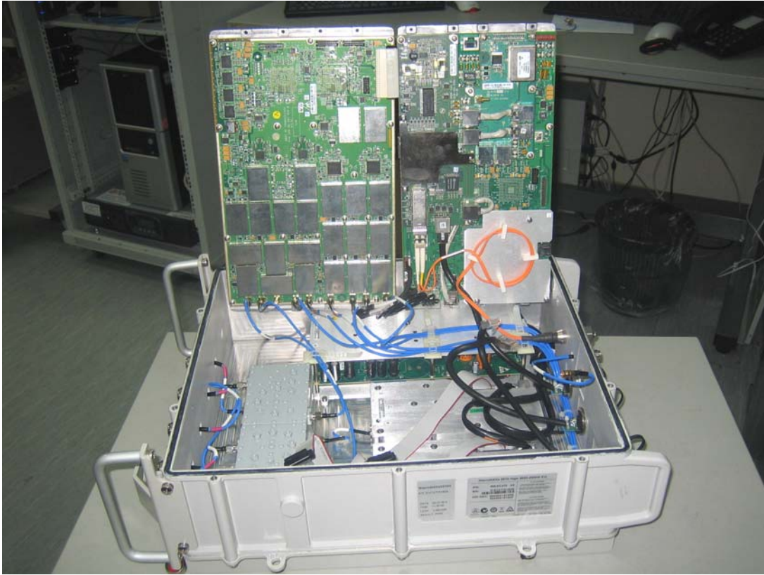
Photograph No.1 “MacroMAXe 2510 Mid” internal view
