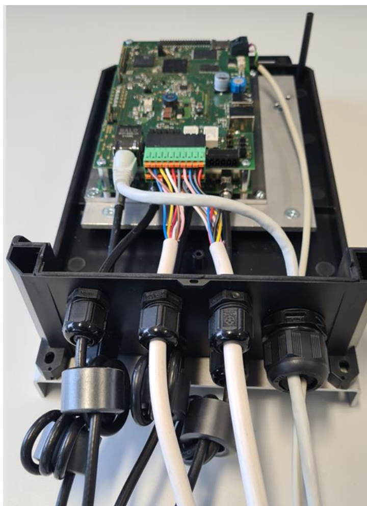
Figure 8: Arrangement of the connecting cables
