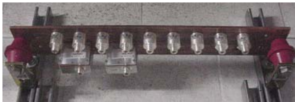
Figure 12: Surge Protectors in Buss Bar (Non-TTA system)
