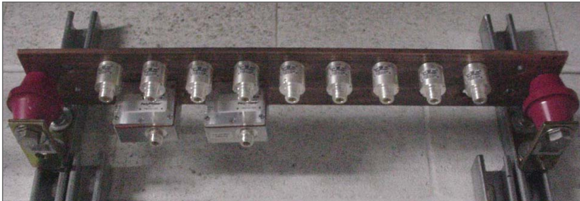
Figure 10: Surge Protectors in Buss Bar
