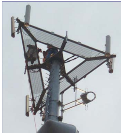
Figure 40: Secured Omni Antenna Mount
