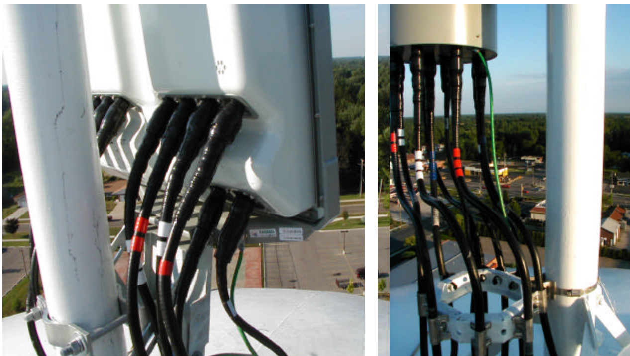
Figure 37: Weatherizing RFS Connectors Cables
