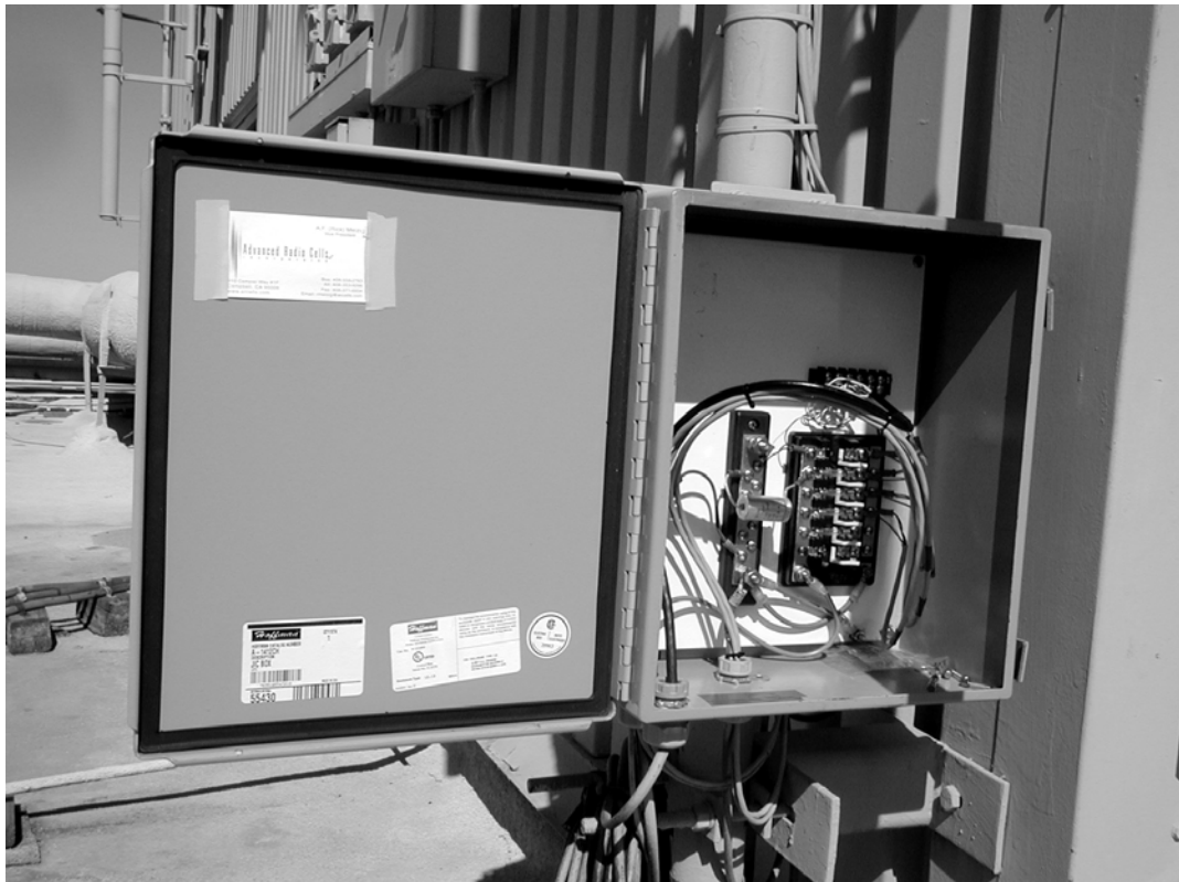
Figure 5-6: Photo of open OJB.
