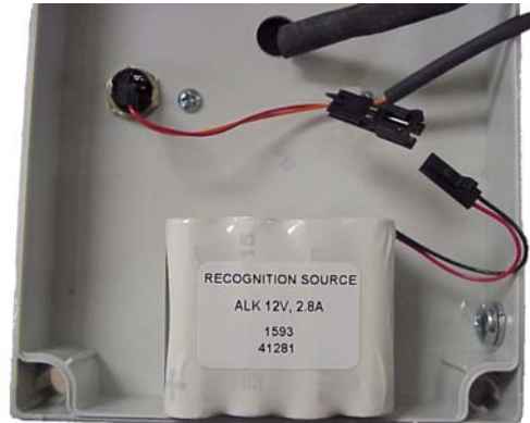
Figure 8-4 – WPR Battery Pack Positioned
