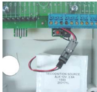
Figure 2-6 – Battery Pack Installed
