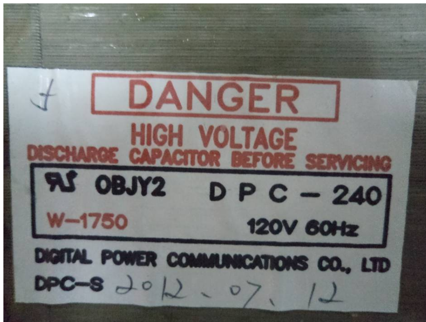
EUT – Power Transformer Label View
