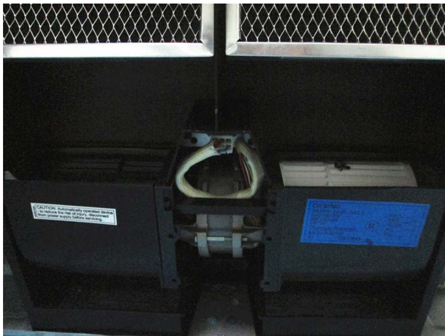
EUT – Exhaust Fans View
