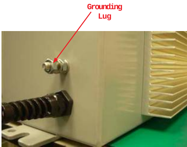
Grounding Lug at Bottom of Wall-mount Chassis
