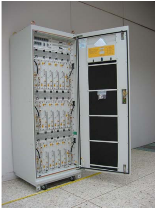
EUT – Inside View (Front)
