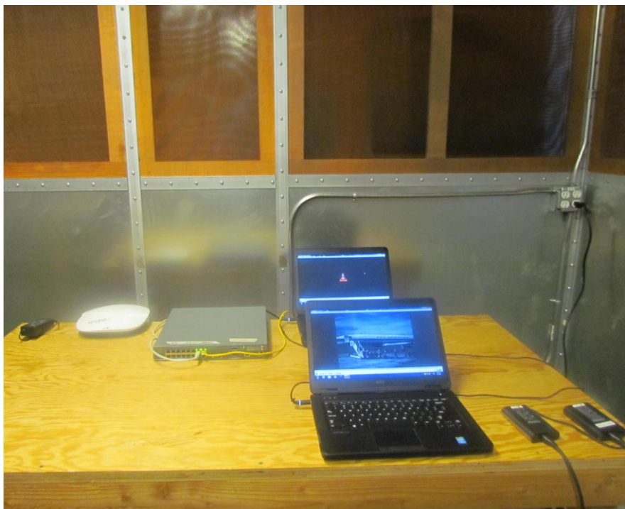
AC DC Configuration Front View
