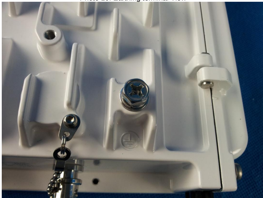
Photo 10. Earthing terminal View
